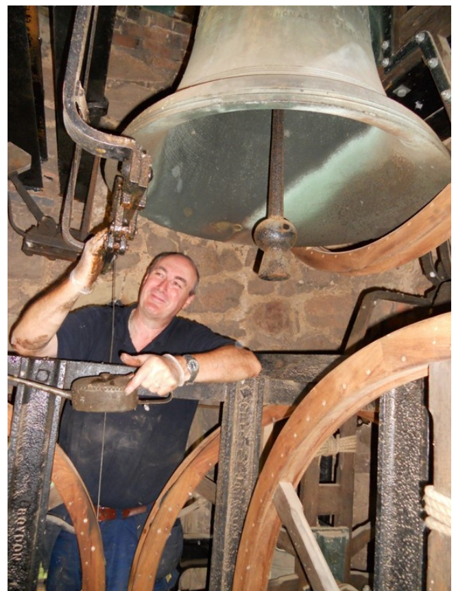
St Peter's 2012 - Brian Johnson, Steeple Keeper, carrying out maintenance on the Seventh bell and stood between the bells on the lower frame
